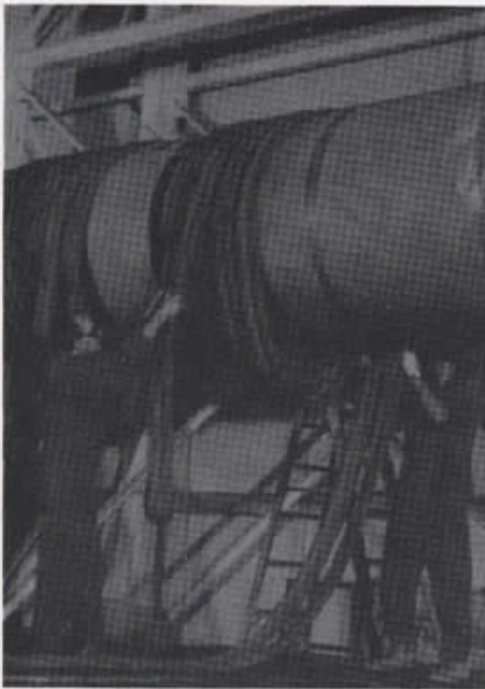
A 100 ton rotor shaft is being rigged for a lift at Ontario Hydro.
